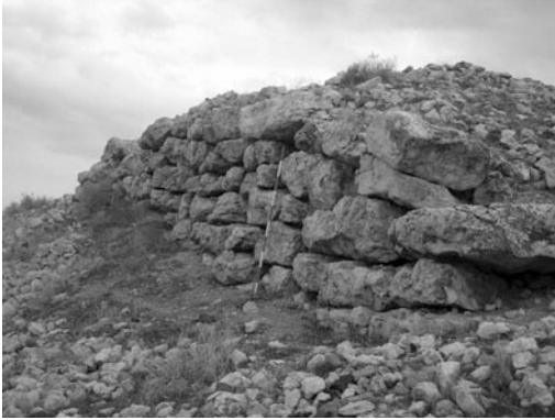
Fig. 10 A view of the defensive wall of the fortress on top of the rock outcrop
